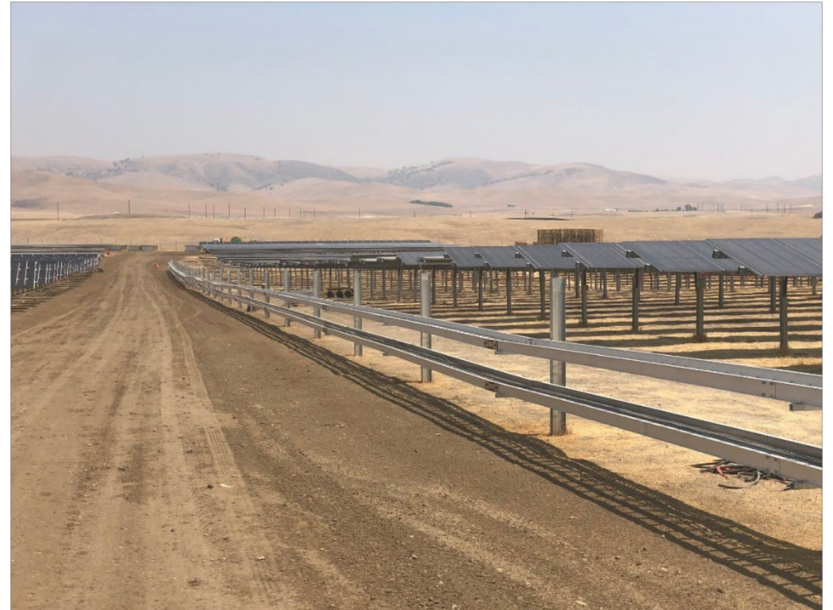
Photo credit: First Solar. Wiring is installed in above-ground trays instead of below-ground trenches
